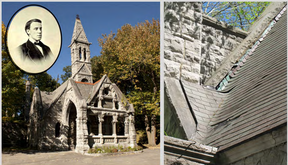
Fig. 5. Designed by architect Joseph Lyman Silsbee (upper left), the mortuary chapel was built in 1879. Over the years the roof joints deteriorated and water was entering the building. To alleviate the problem, flashing at the gable joints was replaced in 2021.
