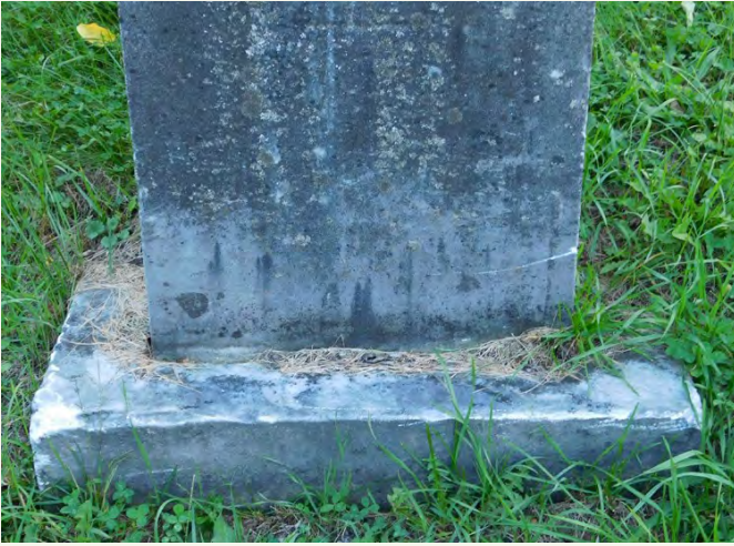
Figure 2. Extensive damage to the base of a marble gravestone from a cemetery Cortland County.
